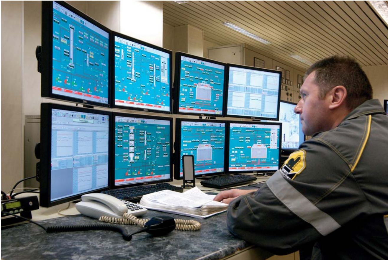
Process control room at Kuibyshev refinery
