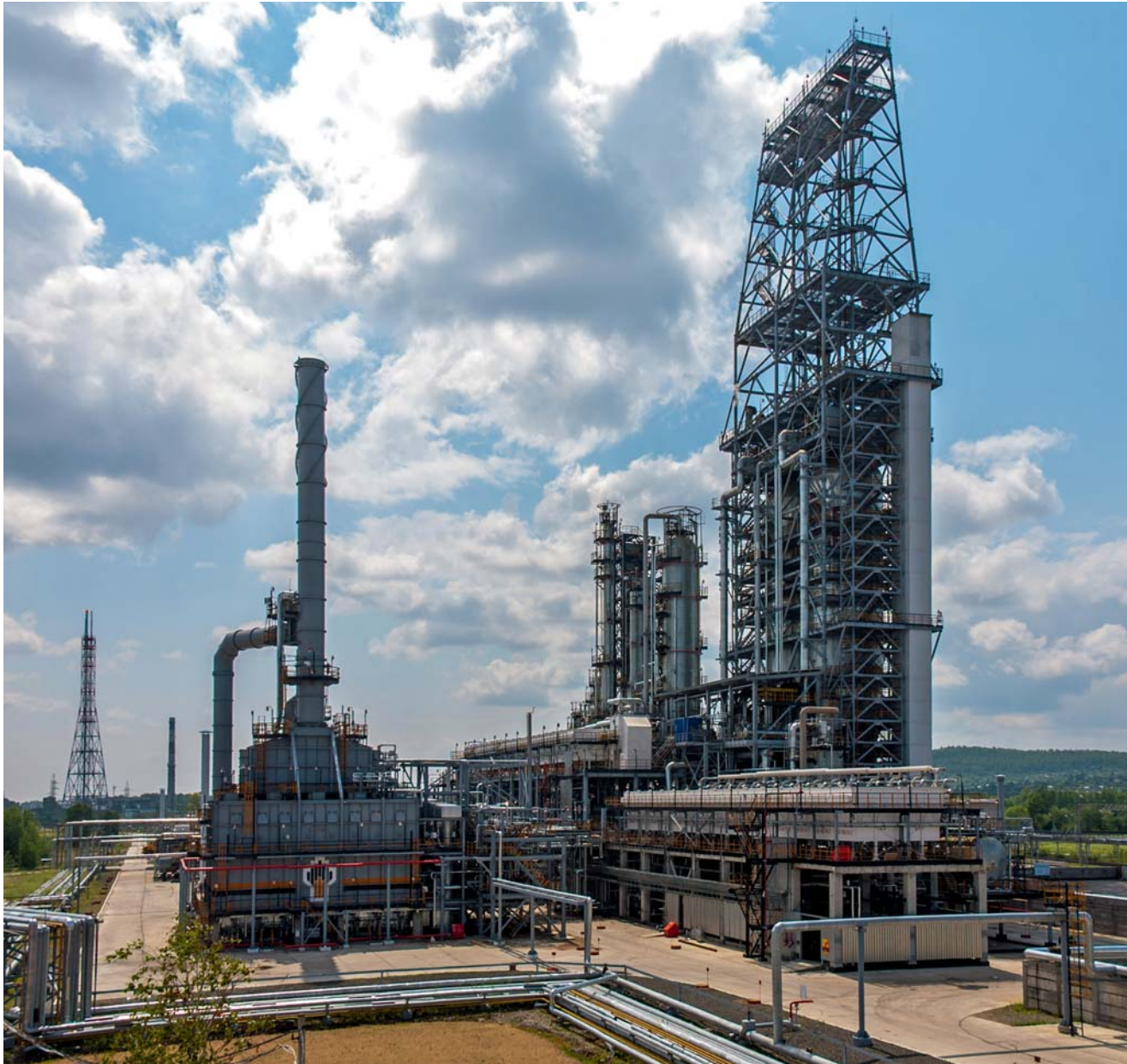
Delayed coking at Komsomolsk refinery
