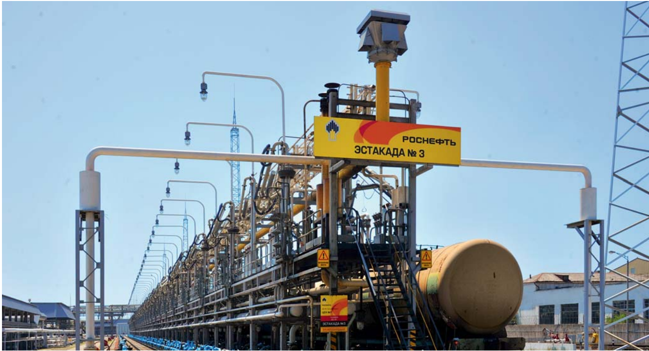
Rack of Tuapsen oil product terminal
