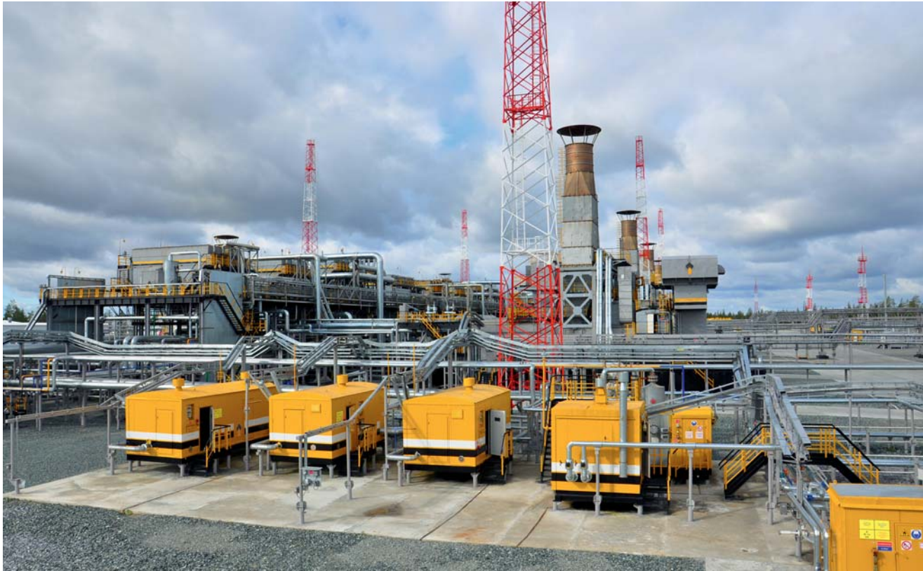
Boosting compressor station at Komsomolsk field
