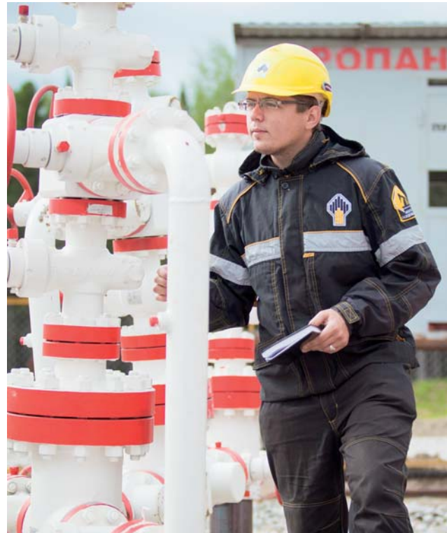
Monitoring of well pumps running
